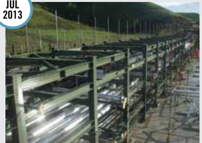
Main pipe rack
